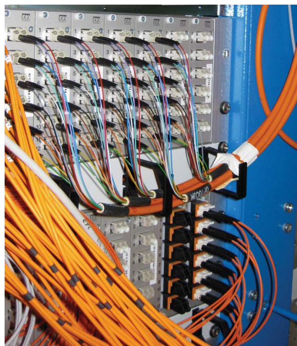
Patch panel with 60 fibres for one TRD supermodule
